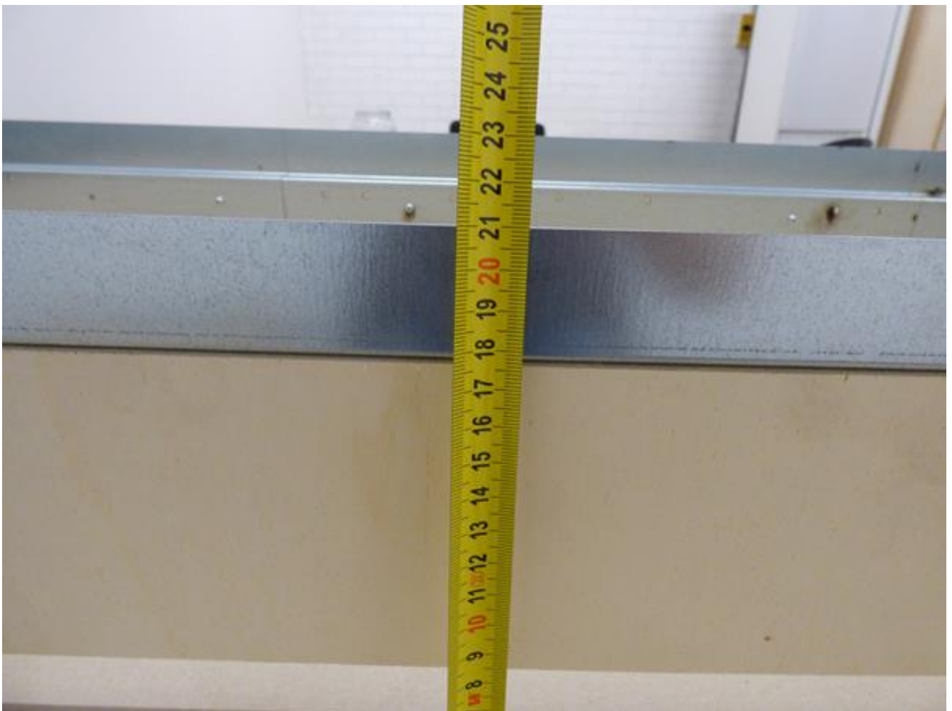
Figure 13 Minimum distance from leading metal edge (surface finish) to the outer wall inside the cavity is 21cm
